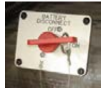
Battery Disconnect Switches
